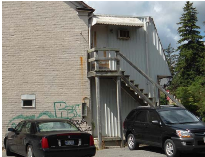
Figure 12: 2 nd floor non-conforming wood exit stair east elevation
