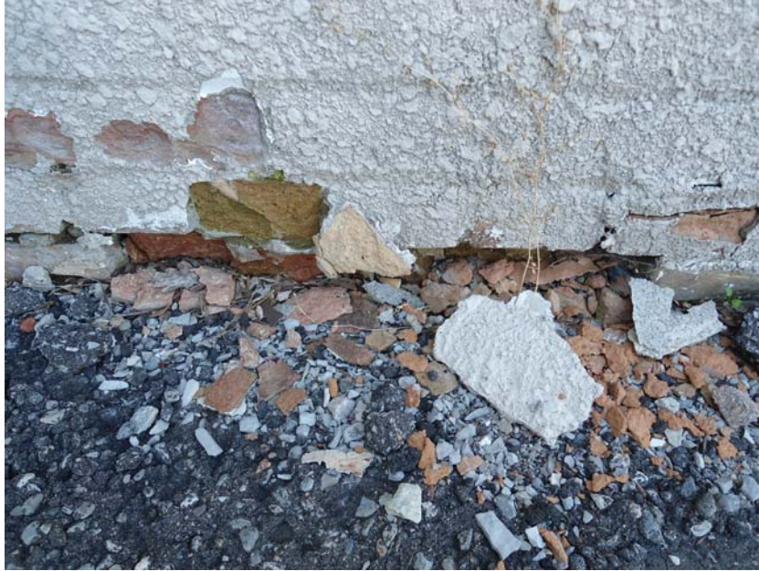
Figure 17: Spalling brick under stucco finish at base of exterior wall
