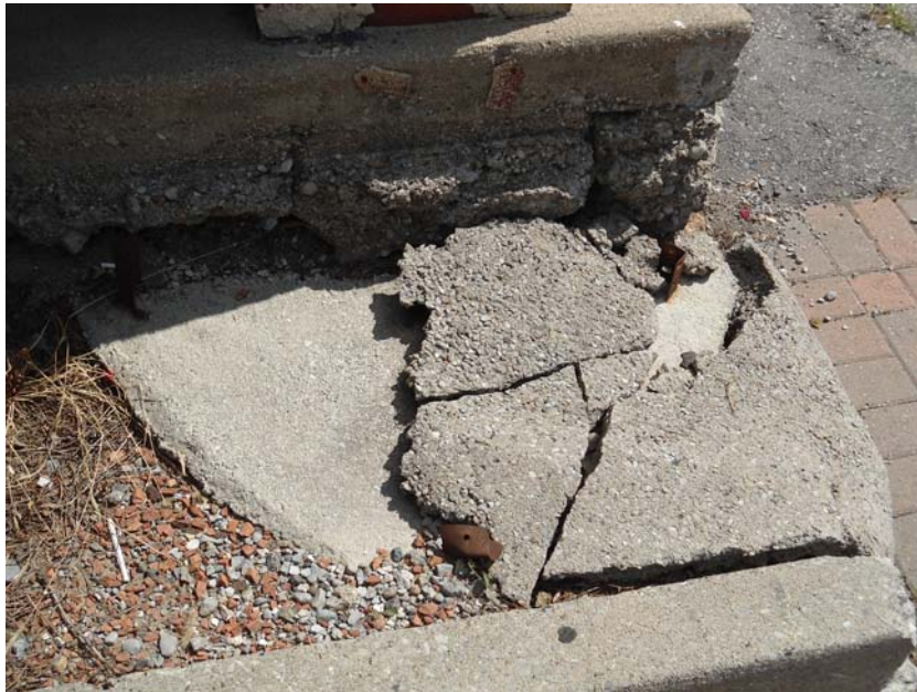
Figure 9: Deterioration of concrete at porch and curb adjacent to public sidewalk.
