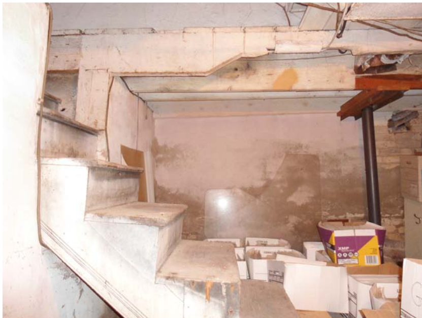
Figure 36: Floor joists cut at stair opening
