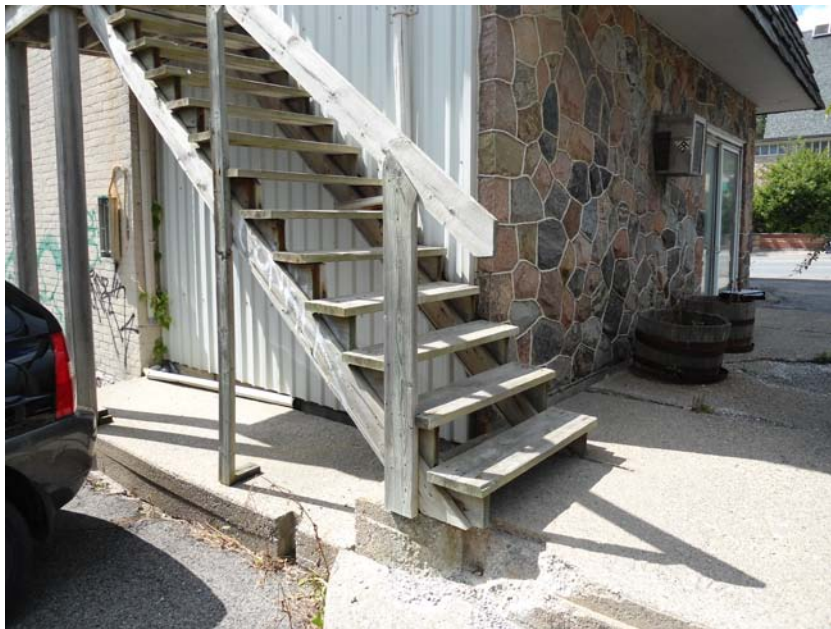
Figure 3: Broken and cracked concrete surfacing. Uneven settlement.
