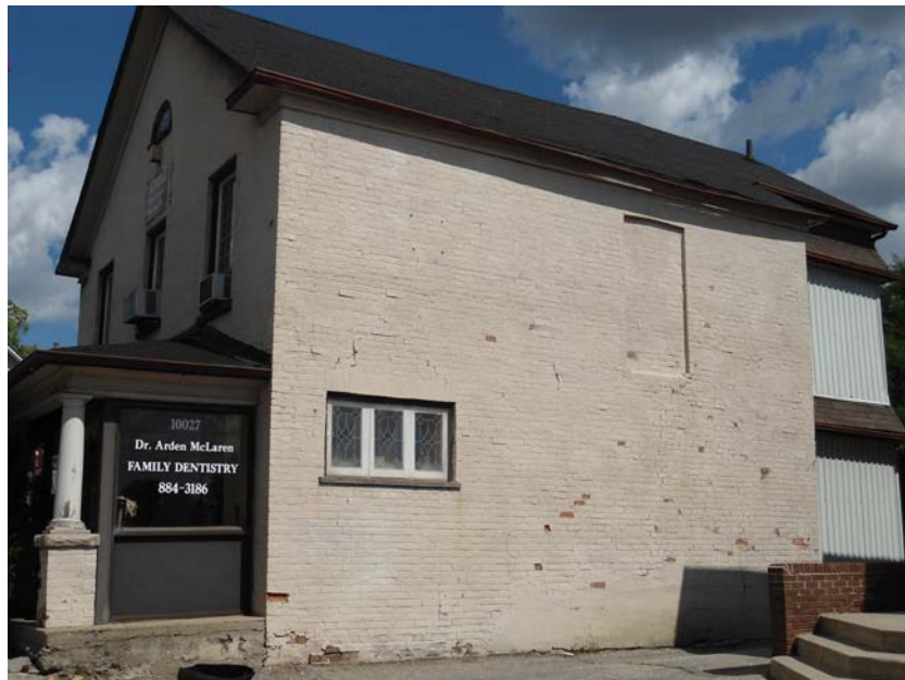
Figure 10: Pronounced sag at roof. Eaves trough bent.
