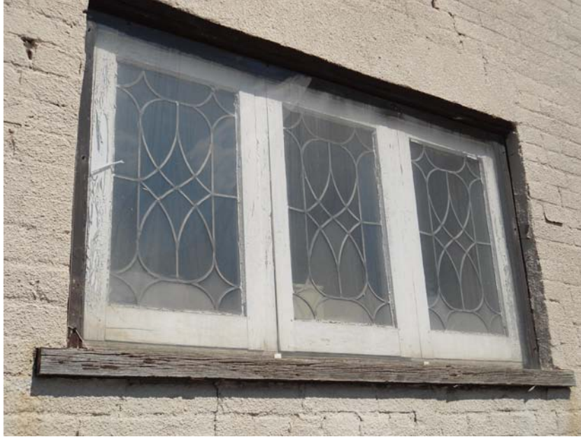
Figure 14: Leaded glass window added at north and south elevation circa early 1900's. Exposed wood sill rotted, plexi-glass fastened over window.
