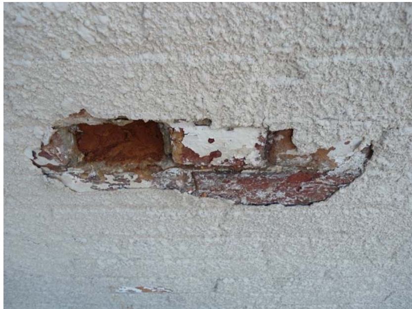
Figure 16: Spalling brick. Previous paint finish exposed by peeling stucco.
