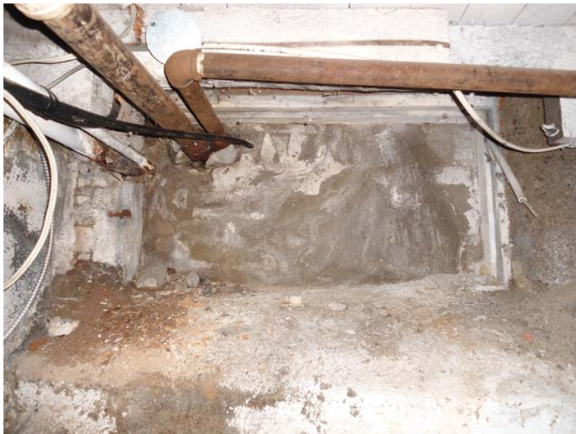
Figure 33: Window at north foundation wall filled with concrete likely at time of 1960's addition
