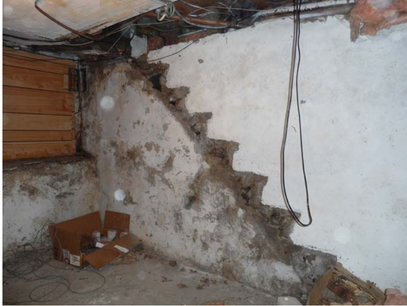
Figure 34: Evidence of stair along east wall removed at time of 1960's addition
