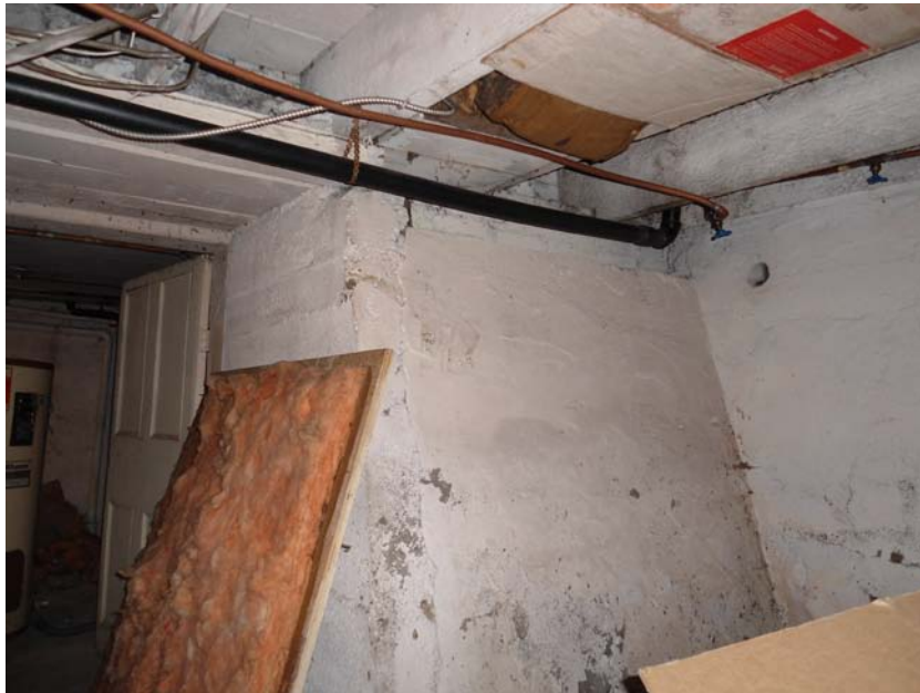
Figure 31: Tapered concrete wall poured adjacent to east foundation wall of original building
