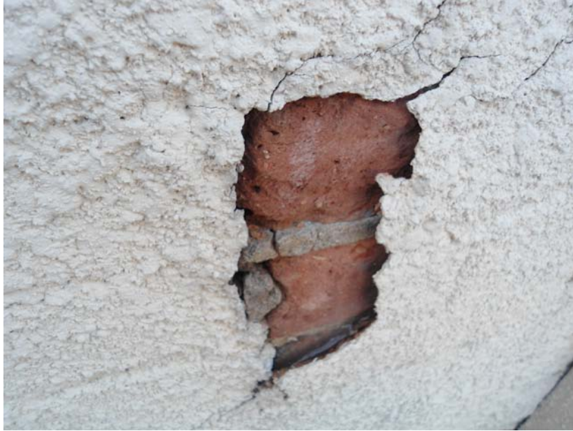
Figure 19: Spalled brick and mortar. Note porousness of bric face.
