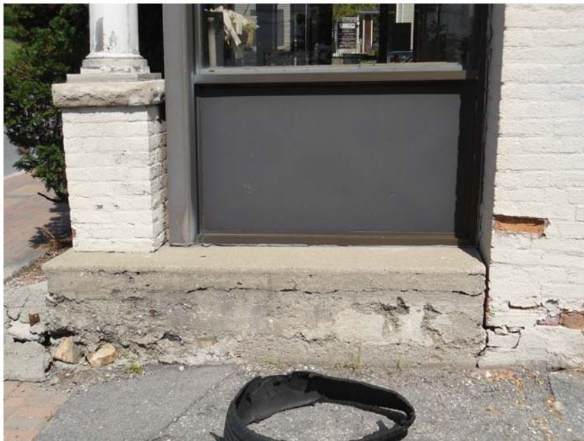
Figure 7: South view of front porch. Concrete disintegrating.
