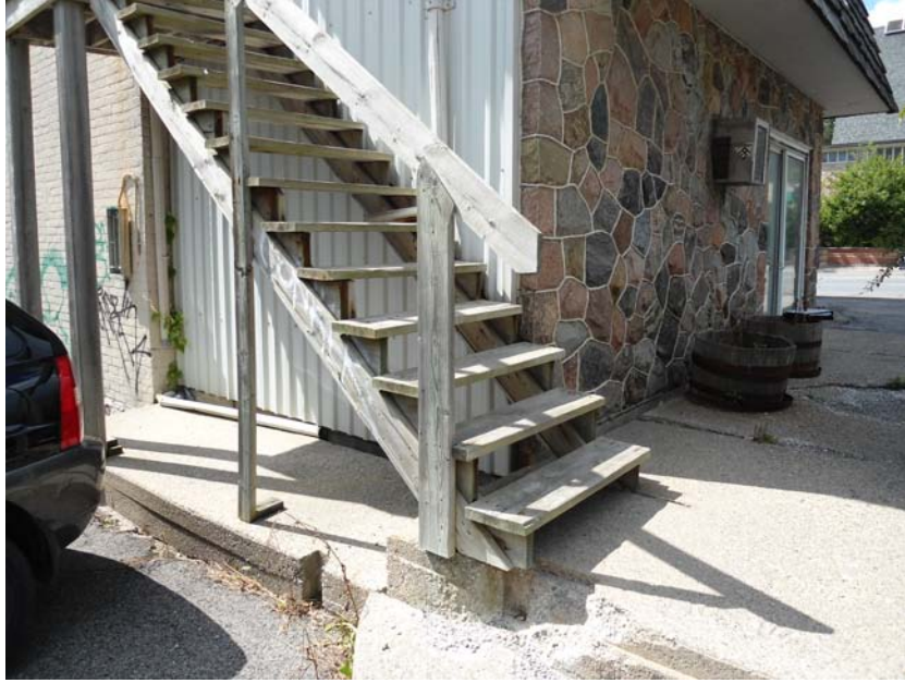
Figure 13: Non-conforming wood exit stair bearing on broken concrete walk
