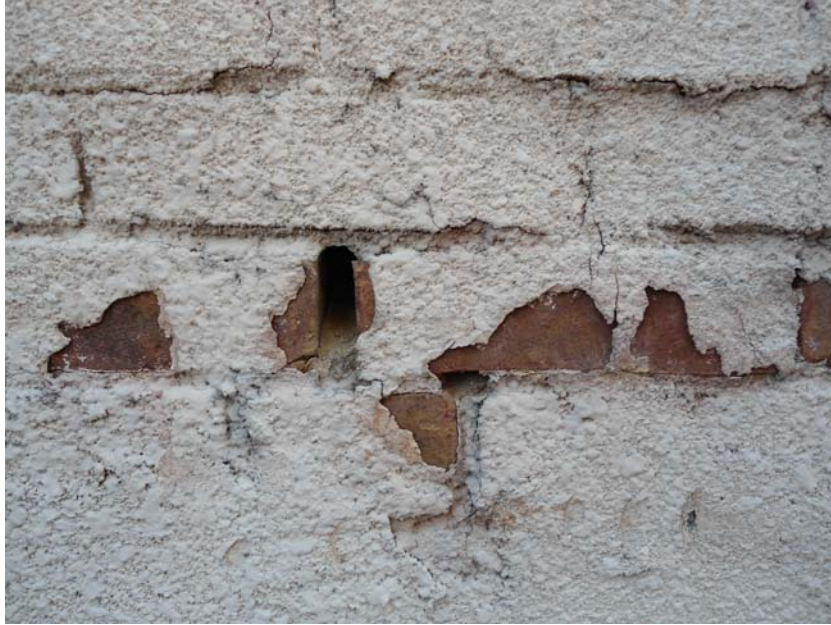
Figure 21: Mortar deteriorated. Remaining dust visible.
