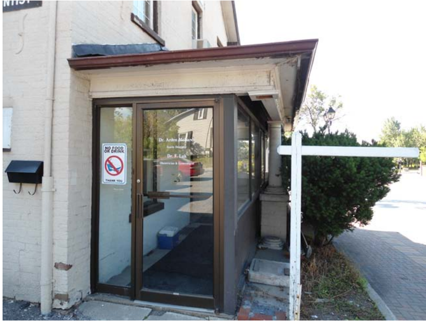
Figure 6: View front porch from the north. missing column, broken concrete at entrance.
