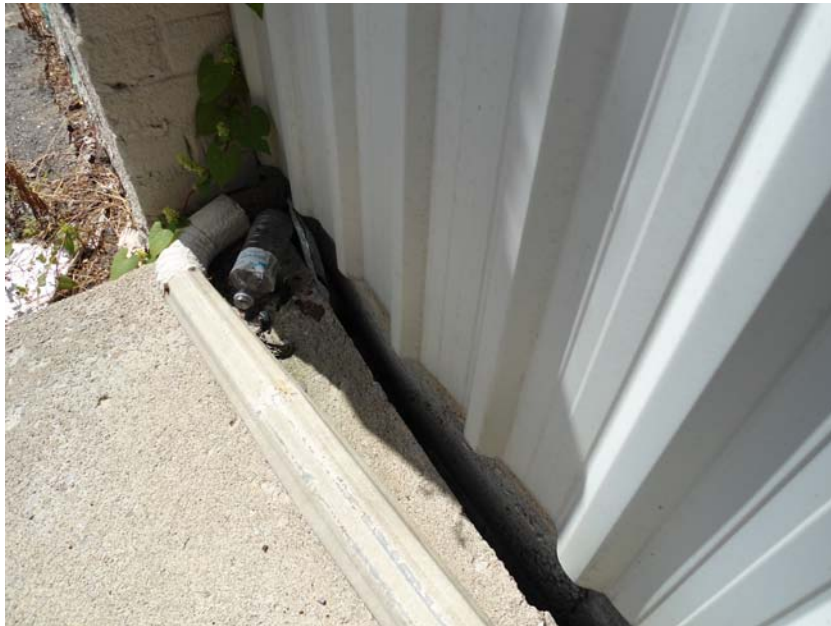
Figure 5: Gap between concrete surface and building. Disconnected downspout
