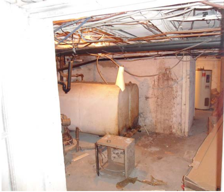
Figure 30: View from original basement through to east addition basement. Note abandoned oil tanks.
