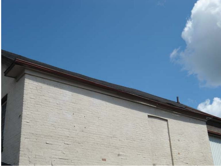
Figure 11: Pronounced sag at roof.
