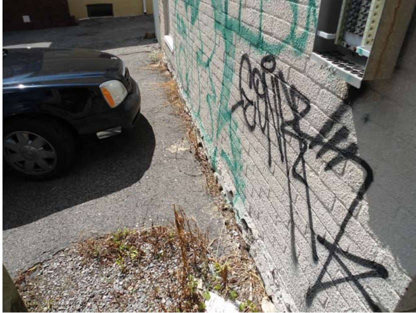
Figure 4: Gap between asphalt and stone foundation at west wall
