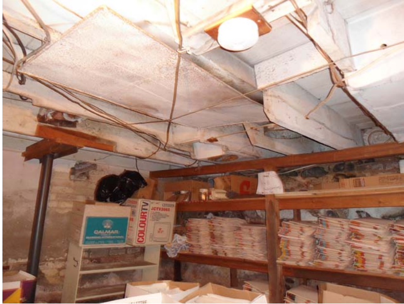
Figure 35: Floor joists under original building have been cut. Note temporary steel post and blocking to support weakened floor.
