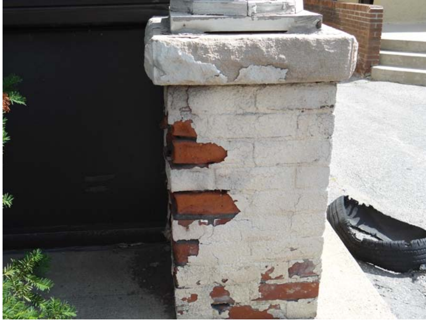
Figure 8: Masonry pier at porch column. Peeling stucco, deterioration of brick and mortar.
