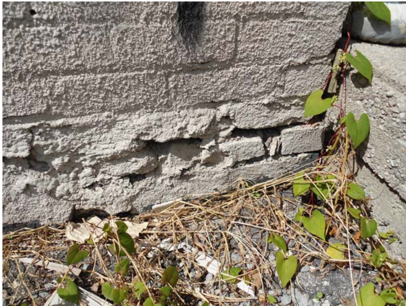
Figure 22: Mortar disintegrated at top of foundation wall
