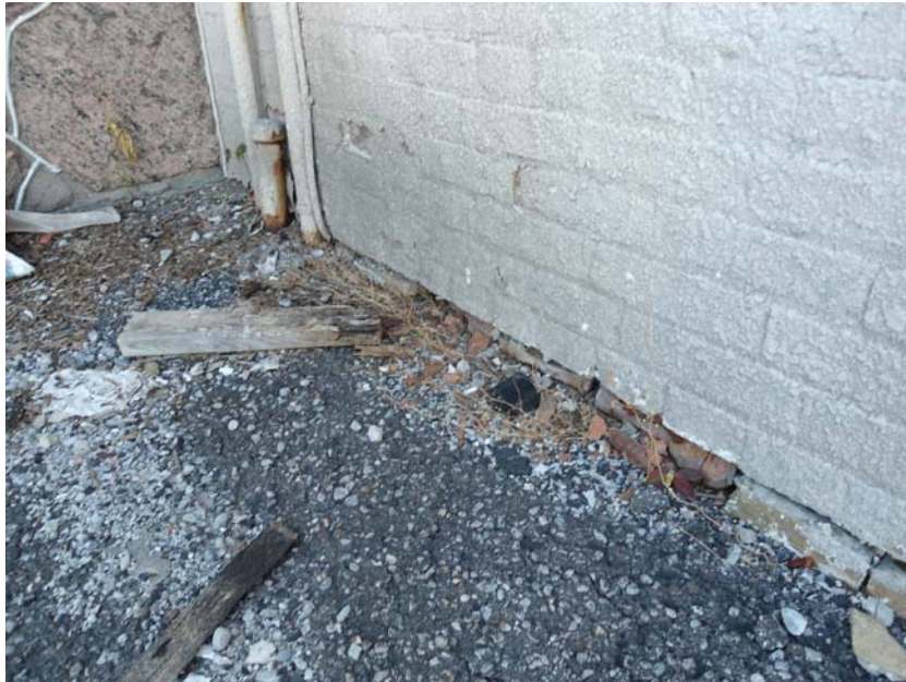
Figure 2: Low point adjacent to north wall of original building
