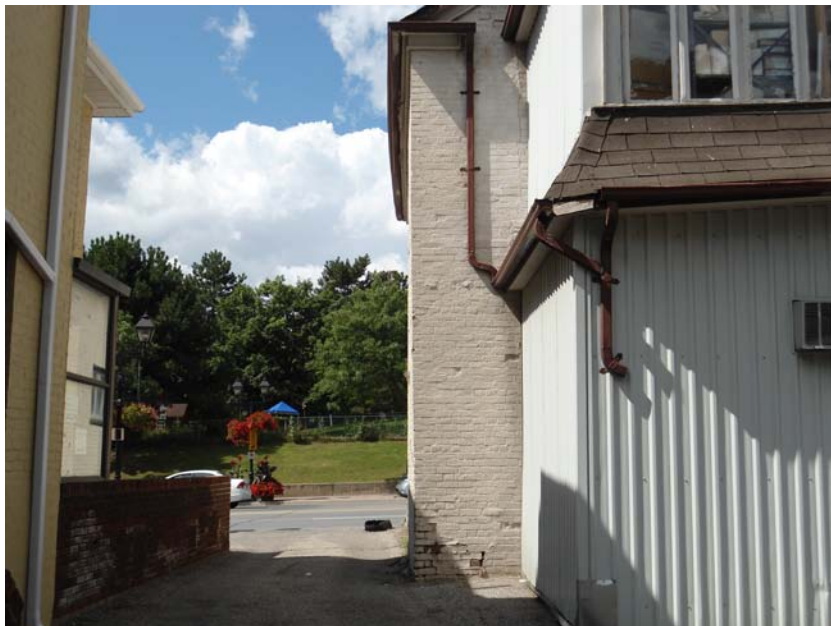
Figure 24: South wall of original building bowed outward.
