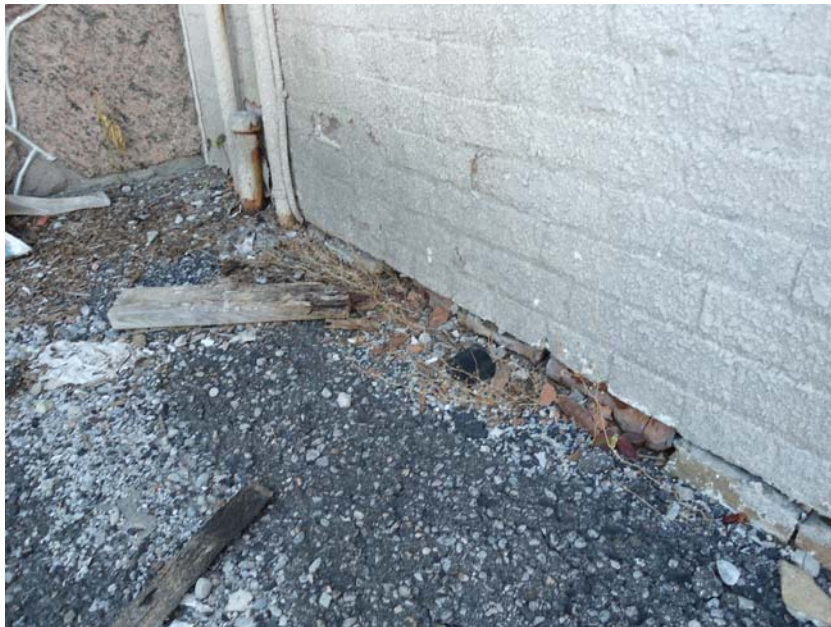
Figure 18: Spalled brick and deteriorated mortar at base of exterior wall. Mortar has completely disintegrated.
