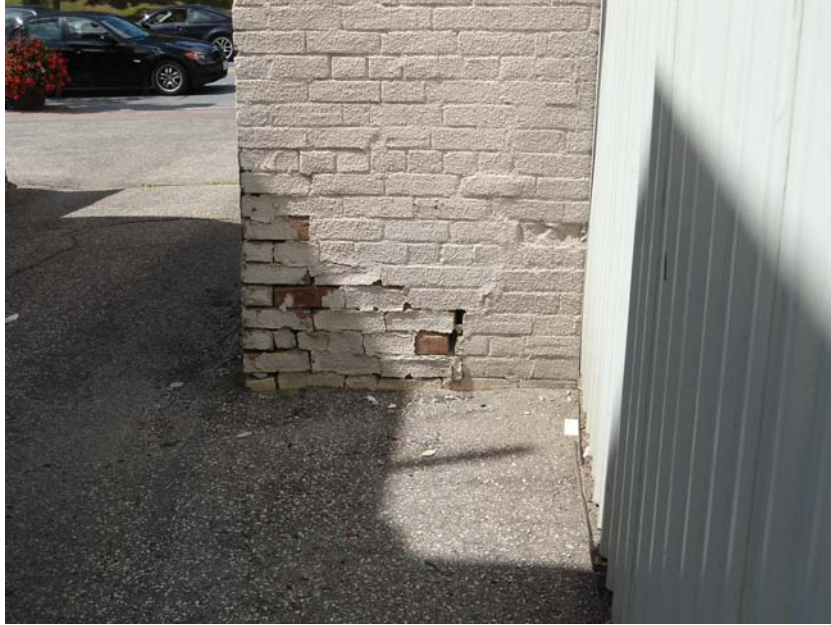
Figure 23: Spalling and missing mortar at base of southeast corner of original building. Base of wall has shifted to the south.
