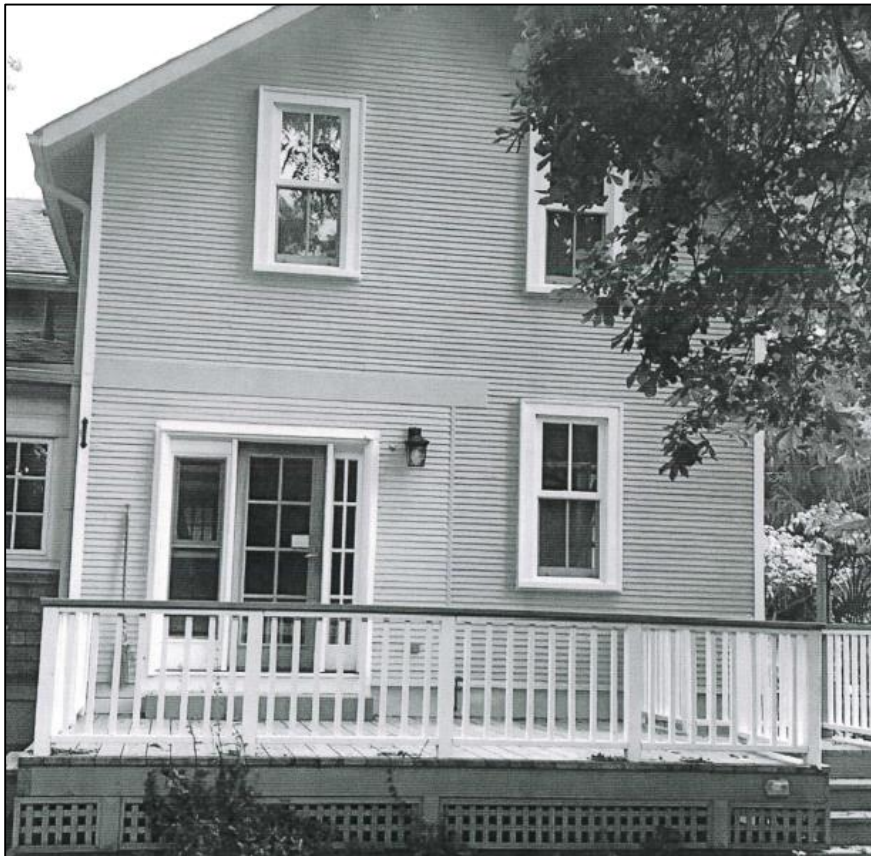
Figure 3: Photo of the McNair-Stallibrass House's rear façade. Note the change in siding around the door, as well as a beam-like element above the door.
