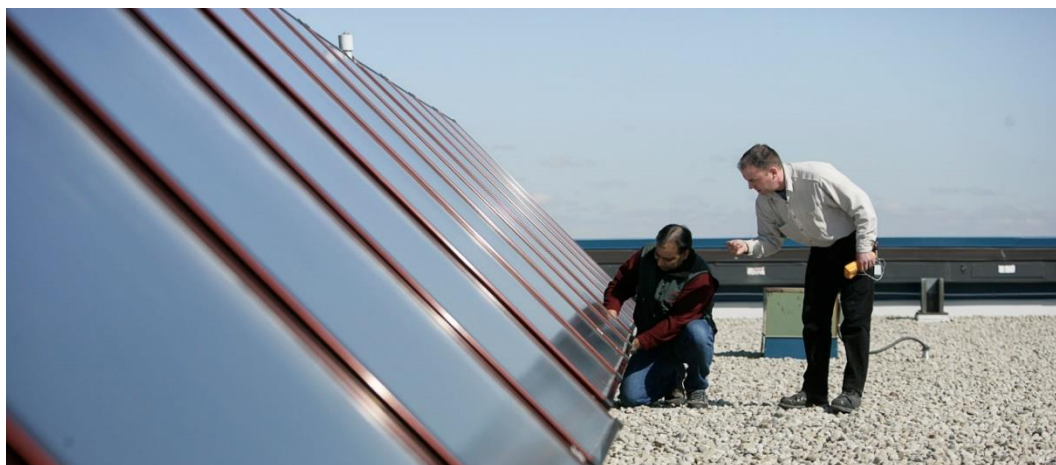
FIGURE 2.5-4 INSTALLING SOLAR PHOTOVOLTAIC CELLS ON THE ROOF OF RICHMOND HILL'S MUNICIPAL OFFICES
