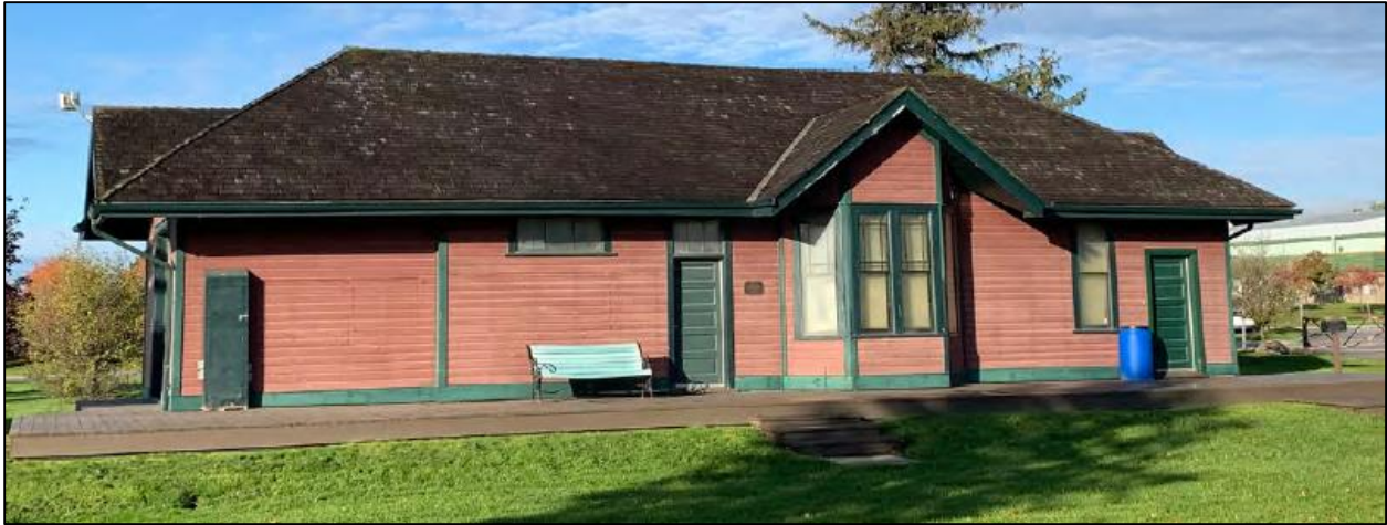
Figure 1: Photograph of the east elevation, showing faded paint and roof shingles that need to be replaced.
