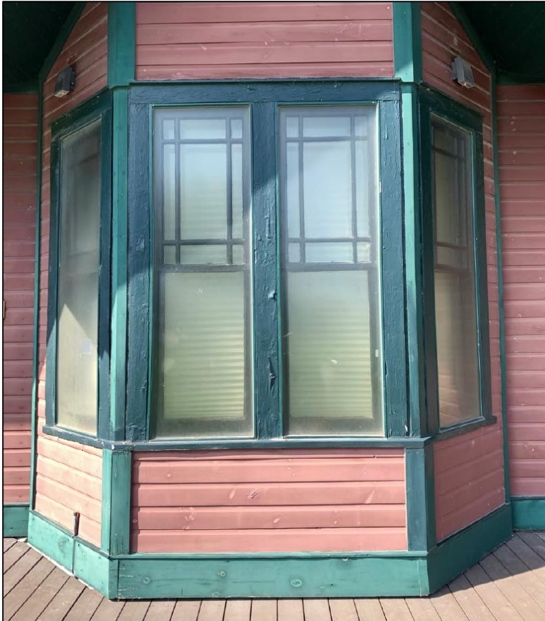
Figure 2: Photograph of a bay window with spalling paint, faded paint, and yellowed plexiglass inserts.
