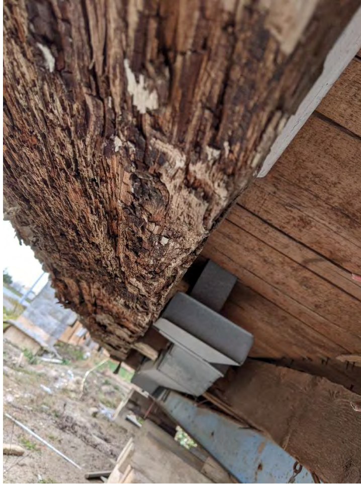
Photo 3. Decayed south sill beam and failed adjacent floor joist.
