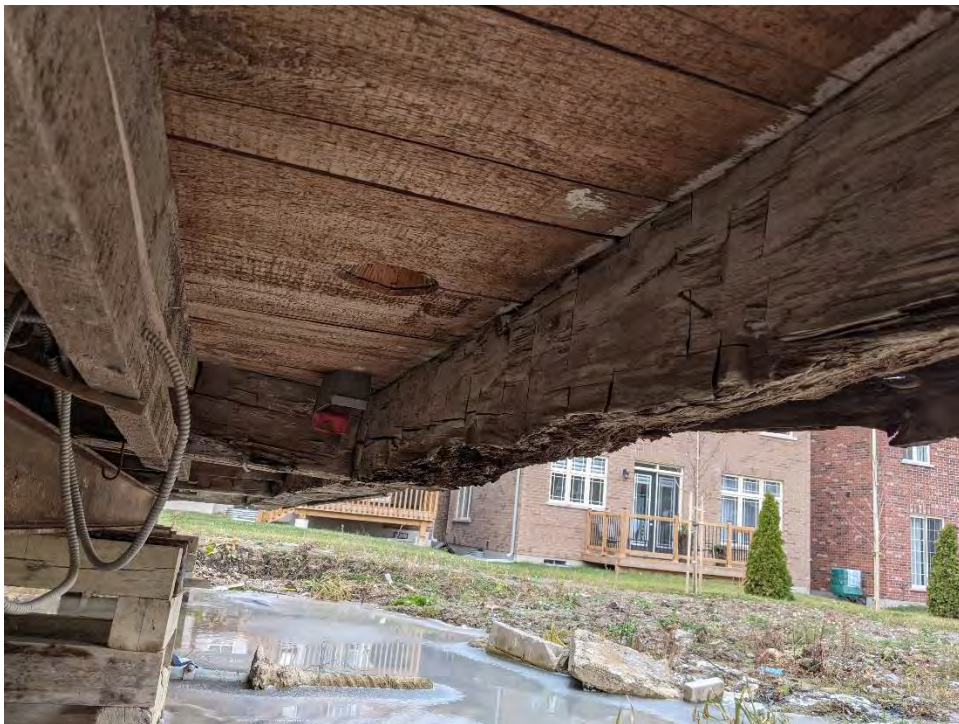
Photo 2. Decayed north sill beam and failed adjacent floor joist.
