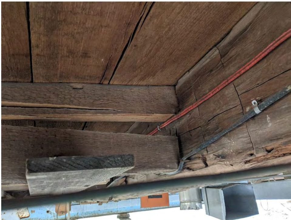
Photo 9. Typical shear failure in floor joist at support. Note decay on underside of intermediate 12x12 beam.
