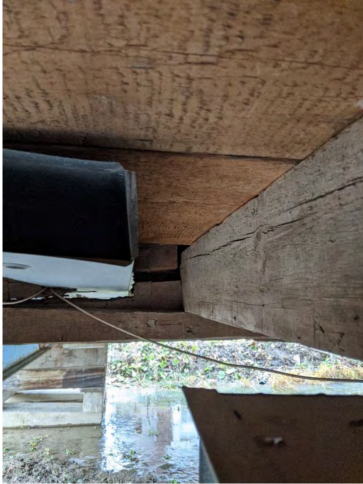
Photo 7. Failed western intermediate beam. Failed at duct.
