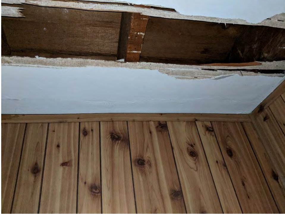
Photo 10. Second floor support structure at north-east corner of ground floor bathroom.
