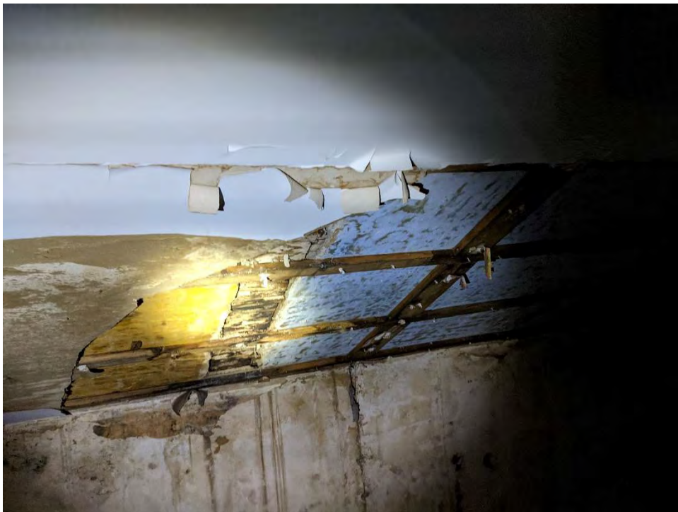
Photo 11. Water damage and mold on lath in bedroom 4.
