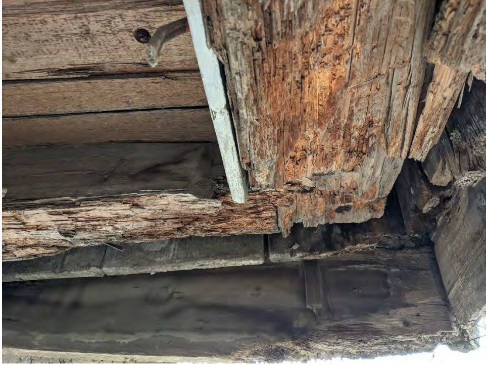
Photo 6. Compromised connection at south-east corner.
