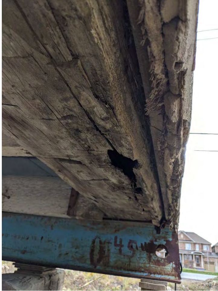
Photo 4. Decayed sill beam at south-west corner of the house.
