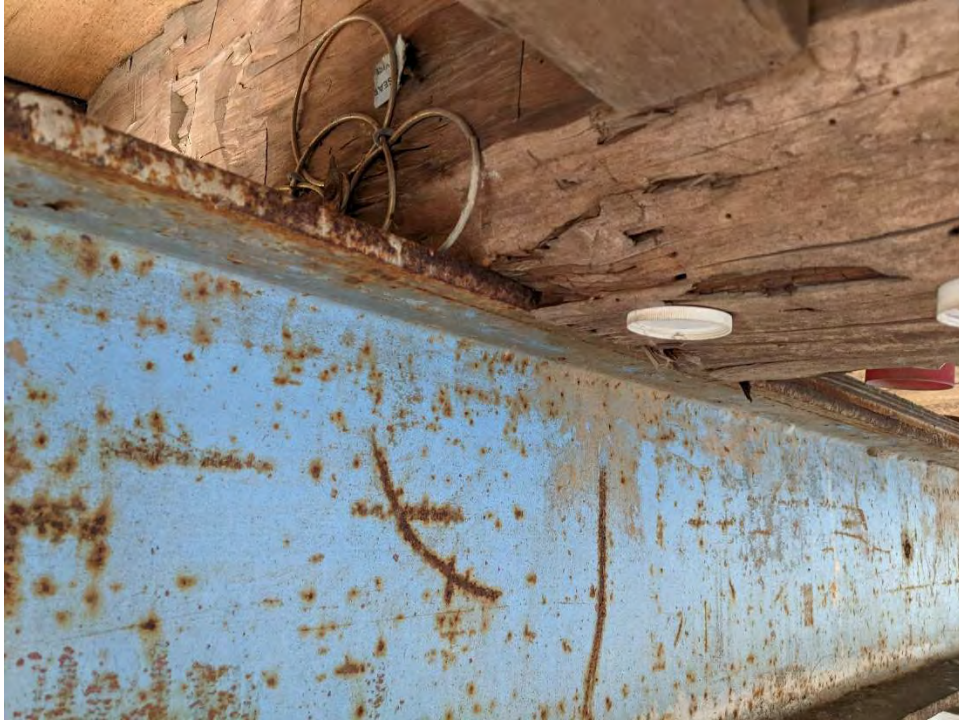
Photo 8. Decayed eastern intermediate beam at south support beam.
