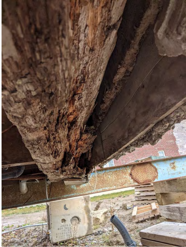
Photo 5. Decayed east sill beam.
