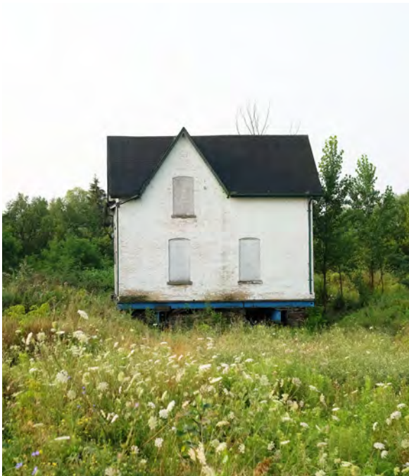
North elevation of the David Hislop House. The structure is currently raised on cribbing (ERA, 2021).
