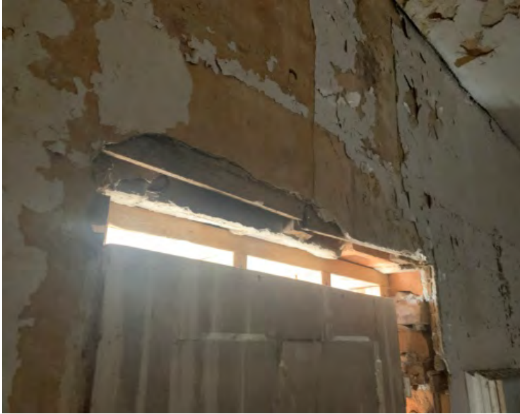
Water damage and build up of mold.
