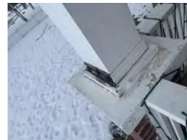
PHOTO 1.2 - REMOVE DAMAGED BASE TRIM AND REINSTALL NEW TO MATCH
