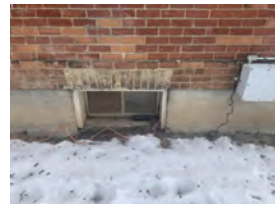
PHOTO 3.1 - WEST BASEMENT WINDOW #1 REMOVE GRADE AROUND BASEMENT WINDOW TO 4" BELOW SILL. REGRADE AREA TO SLOPE AWAY FROM BUILDING. REPLACE CONCRETE SILL. REPAIR WOOD FRAME. REPAINT AS REQUIRED.
