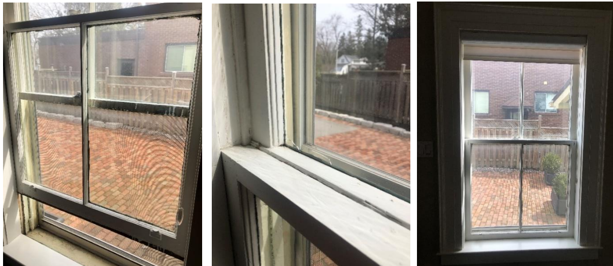
Figure 5 Photographs showing typical existing wood windows at 210 Richmond St., to be replaced with new wood window units to match the existing.
