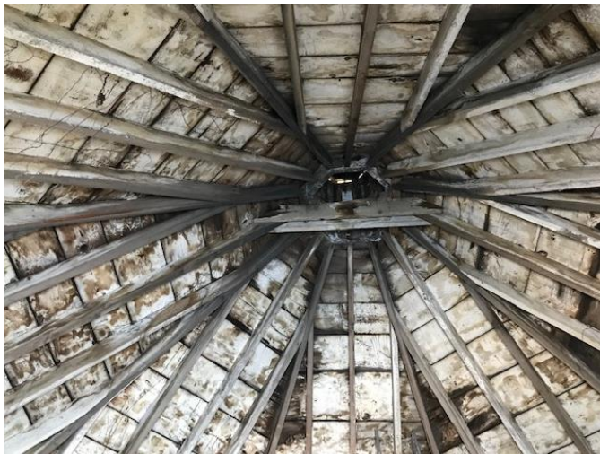
Figure 4 View of the Vault rafters and roof deck. The roof structure, though stained and damp due to the leaking roof finish, remains firm and undecayed (source: Edwin Rowse Architecture Inc.).
