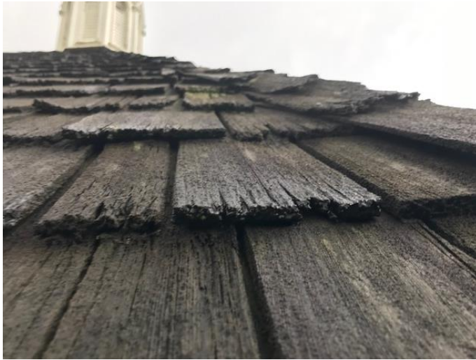
Figure 3 Detailed view of the Vault's existing deteriorated roof shingles (source: Edwin Rowse Architecture Inc.).
