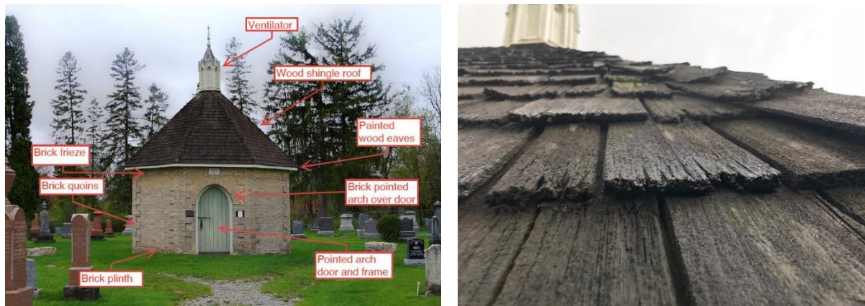
Figure 2 Image showing the Octagonal Vault's architectural elements (left), and a detailed view of the building's existing highly deteriorated wood shingles (right), which are proposed to be replaced with a new asphalt roof.
