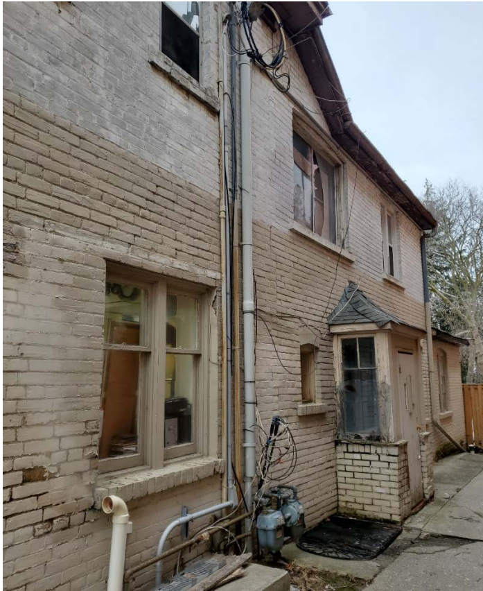
Figure 6 Current photograph looking northeast, showing the south elevation of 10217 Yonge Street. Note the wooden window units and brick lintels and sills. (Source: HUD, 2024)
