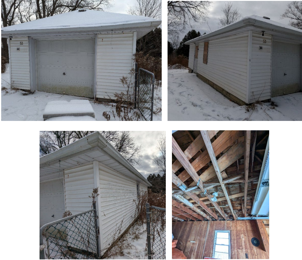
Figures 27-30: Views of the exterior and interior of the detached garage. (MHBC, 2024)
