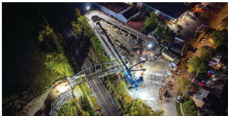
Construction of the Pedestrian and Cyclist Bridge at David Dunlap Observatory Park
